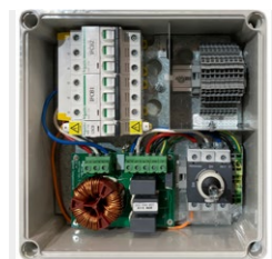
Ebox Wiring Integration
