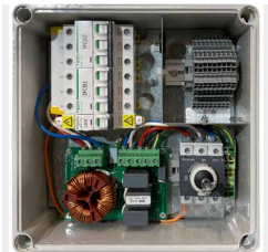
Ebox Wiring Integration
