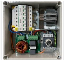
Ebox Wiring Integration
