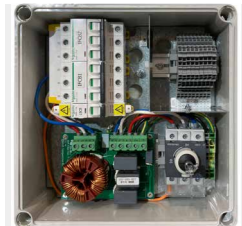
Ebox Wiring Integration
